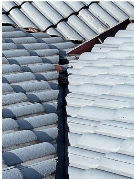
Photo Ref #54: There are several valley tiles that have moved out of alignment. This should be re-aligned to prevent possible blockage and/or
