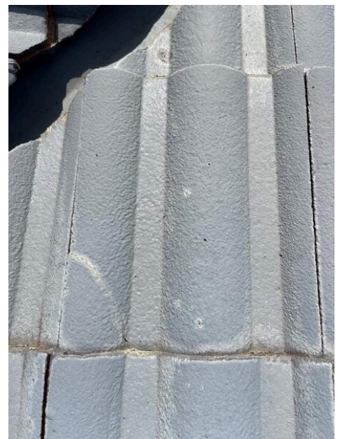
Photo Ref #47: There are several repaired cracked tiles to the roof exterior. This should be monitored as silicon will deteriorate
