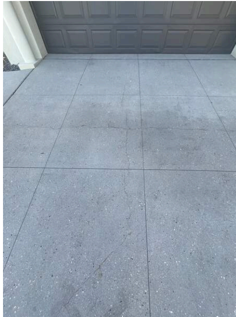
Photo Ref #41: There is moderate cracking to the concrete driveway. This should be monitored for further cracking
