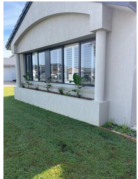
Photo Ref #19: The external garden bed level is higher than the bedroom four internal floor level suggesting possible lateral dampness
