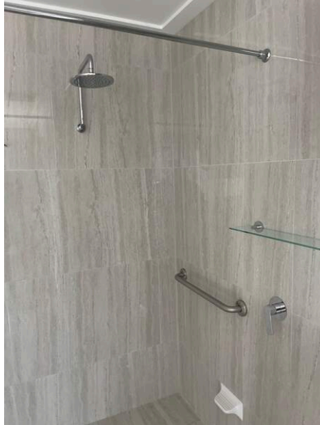
Photo Ref #13: There is moderate water hammering to the ensuite taps. This will require a licensed plumber to inspect and assess.
