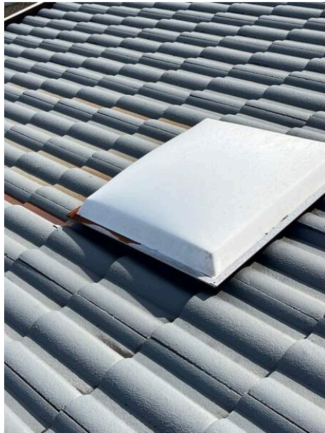
Photo Ref #52: There is moderate corrosion to the skylight structure
