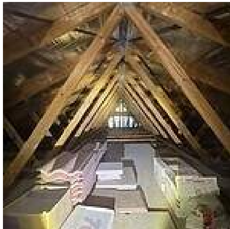
Photo Ref #30: The roof trusses have been incorrectly loaded for storage. Trusses should not be loaded on the webbing and bottom cords.
