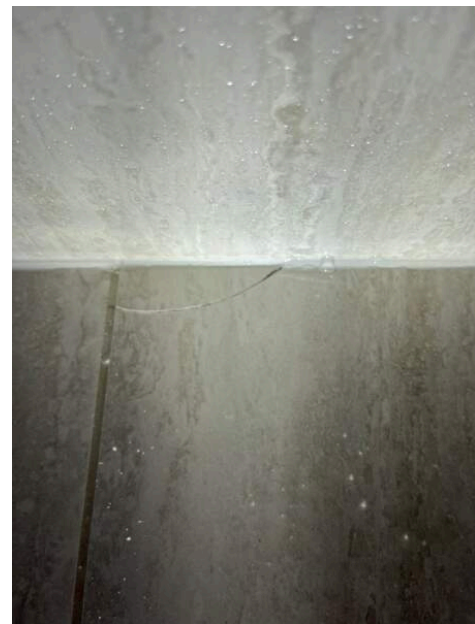
Photo Ref #12: There is a cracked tile on the shower floor. This should be repaired/renewed to prevent possible moisture ingress into the substrate.
