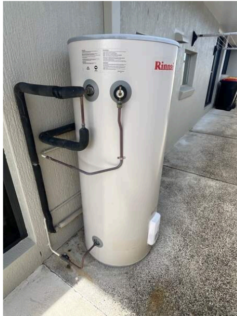
Photo Ref #26: The hot water system is an electric hot water unit. There were no visible defects to the hot water system on the day of inspection
