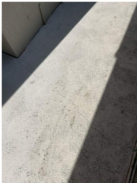
Photo Ref #42: There is moderate cracking to the eastern concrete path.
