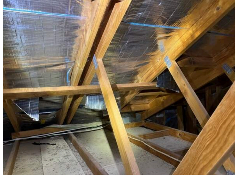
Photo Ref #31: The sarking is torn in several areas. The affected areas should be repaired to prevent possible moisture ingress.
