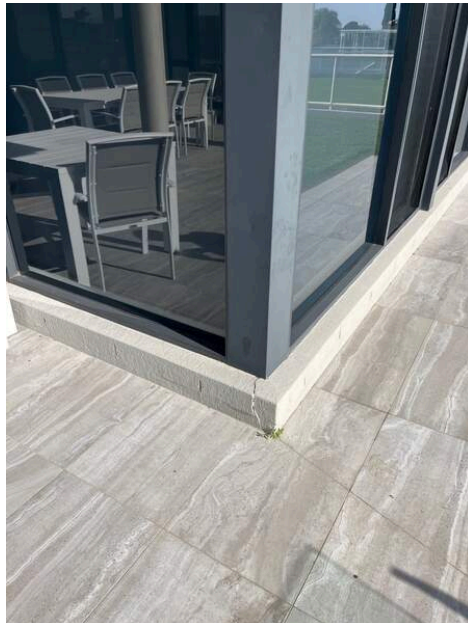
Photo Ref #37: There is moderate cracking on the lounge room rear windowsill. This should be repaired to prevent moisture ingress into the surrounding areas
