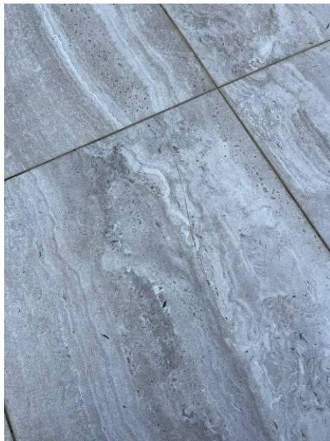
Photo Ref #7: There is a cracked tile on the front entrance floor
